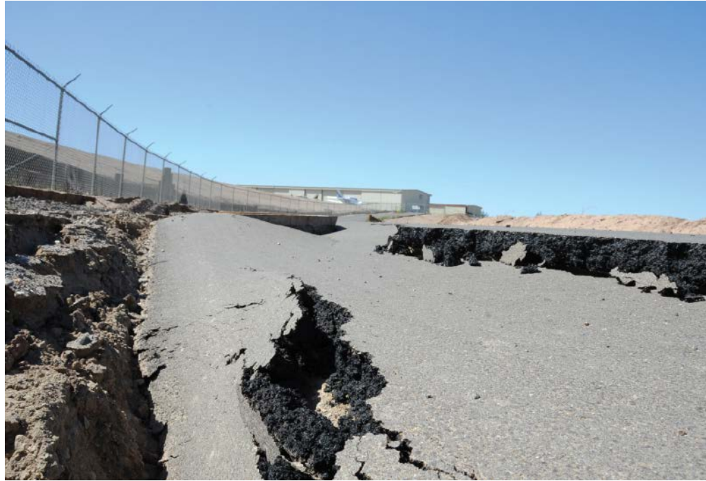
A magnitude 7.2 earthquake damaged roads across northwestern Mexico and Southern California, like this one in Calexico, when it struck on 4 April 2010. Credit: Adam DuBrow/FEMA
