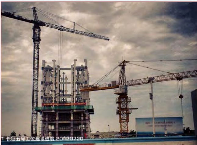
Wenchang construction progress: the launch tower is taking shape. (credit: Chinese Internet)
