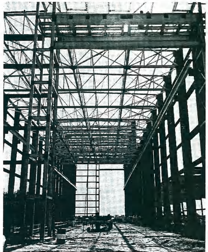
STEEL LACEWORK of MSC's Operations and Checkout Building at the Merritt Island Launch Area, provides artistic view to ground-level observers. Construction on the $7.6 million facility is progressing rapidly.
