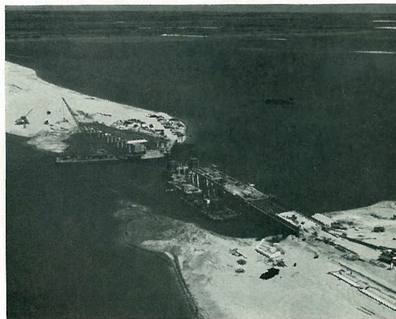
DIVERS are at work just to the left of the Banana River-Orsino bascule bridge, above. Water is 20 feet deep in the channel.
