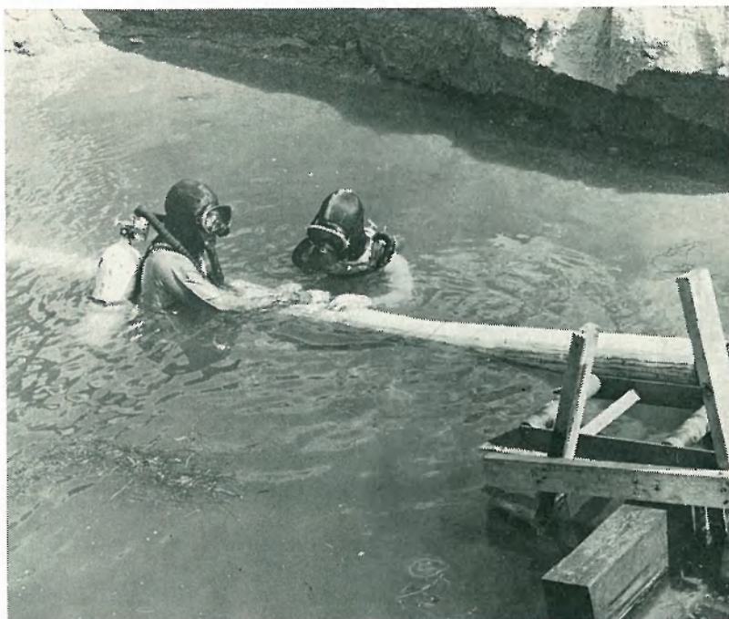
DIVERS Bill Sproul, left, and Buddy Thompson inspect pipe as it is lowered into the Banana River. They have been working 20 feet deep, installing the pipes in underwater trenches.
