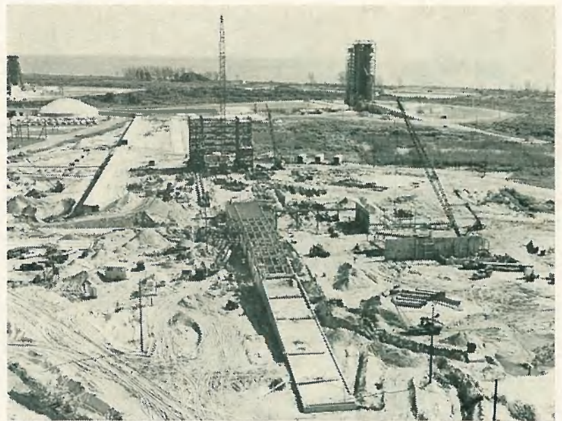
AERIAL VIEW of Launch Complex 36, looking east, shows construction progress of Pad A, service structure and access ramp. Pad B is in background.
