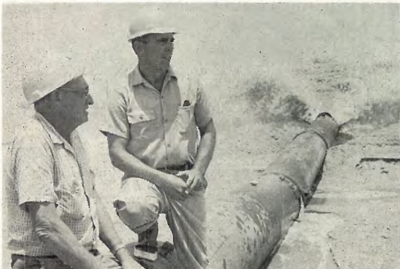
DUMP SUPERINTENDENT Joe Miller, left, and Wally Ericson take a minute's break as river bottom pours through pipe into a fill area.
