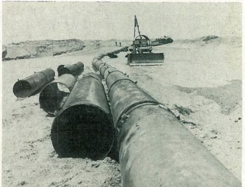
FILL HAS BEEN used to mold the crawlerway and an 80-foot mound of surcharge at Complex 39's Pad A. Four stockpiles have also been set aside for future use.
