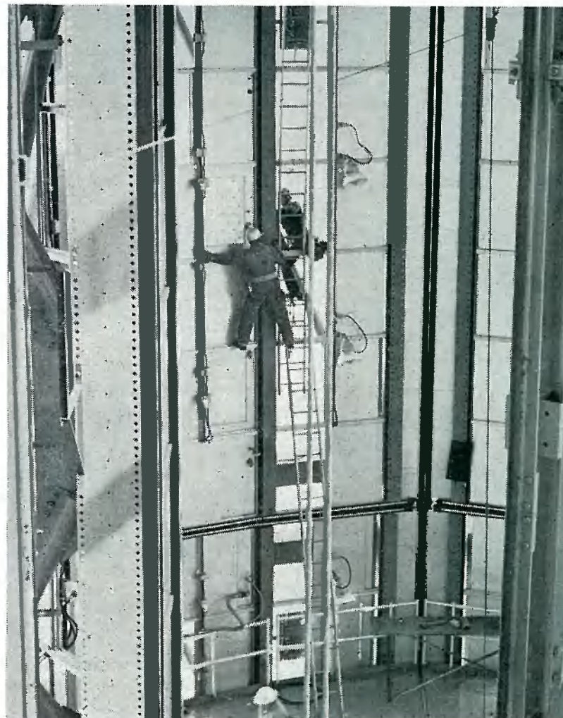
INSIDE the silo gates that adjoin 37's service structure, two electricians check out newly-installed wiring.
