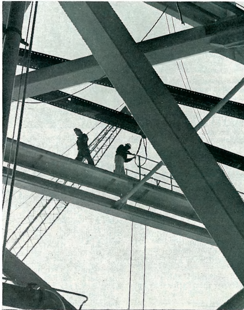
FRAMED by steel patterns high up in Launch Complex 37's service structure, two workmen busily go about their business. For the up-to-date story and photos on construction progress, turn to Page 4.
