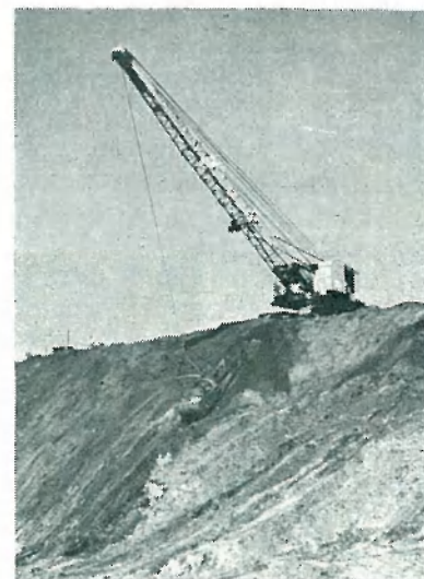
SIDES OF 35-foot mound are smoothed from the top by dragline and bucket. Dirt was carried from borrow pit up incline to the top of the mound by huge but fast rolling earth-moving equipment.
