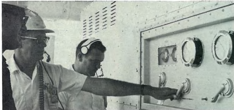
G. L. STEINES, K. C. Jordan and C. H. Ormond, all of Chrysler, run air conditioning checks on environmental control system.
